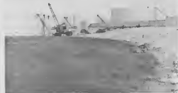
Because of heavy coral rock formations, dynamite blastings are necessary to level off this area which is reserved for Jet Fuel tanks.
